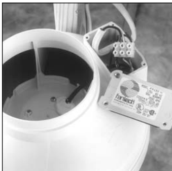
Romex wiring – Top View
